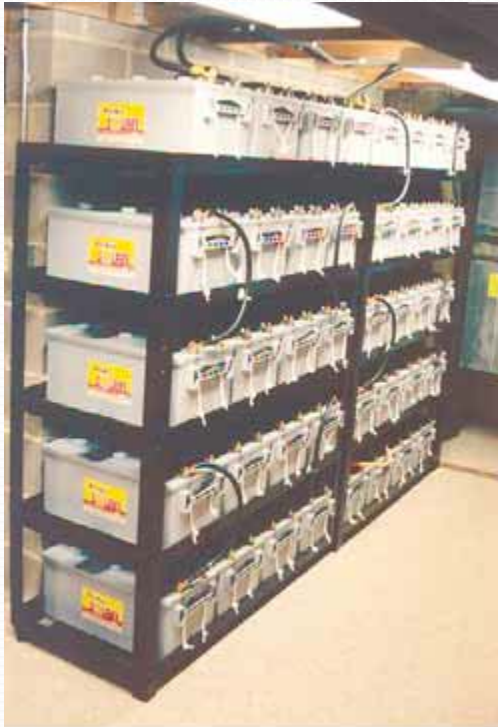
Sealed solar gel batteries located in an open basement rack
